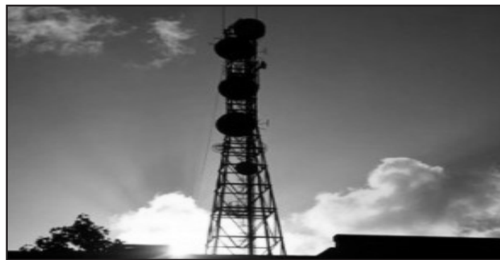
Figure 3 : A Base Station
